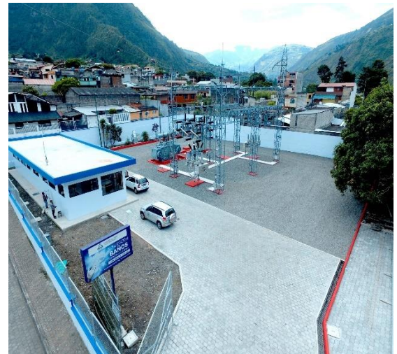
Figura 7 Subestación Baños - Tungurahua-Ecuador https://www.eeasa.com.ec/content/uploads/2021/11/DJI_0014.JPG-2048x1536.jpg
