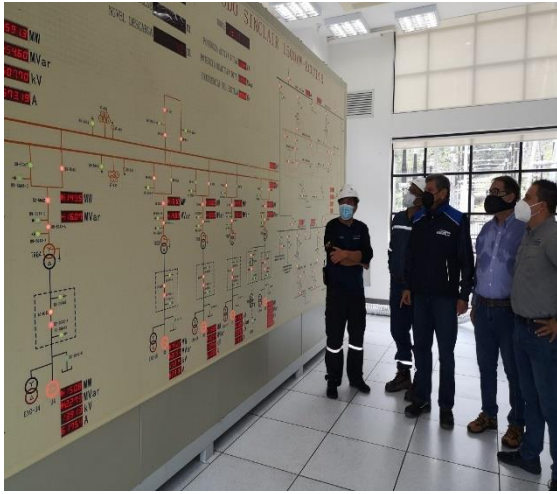
Figura 8 Sala de Control de la Central Coca Codo Sinclair https://www.celec.gob.ec/hidroagoyan/wp-content/uploads/2021/11/CCS_100.jpg
